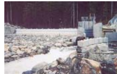
Run of River Bypass & Gate Chmbr
